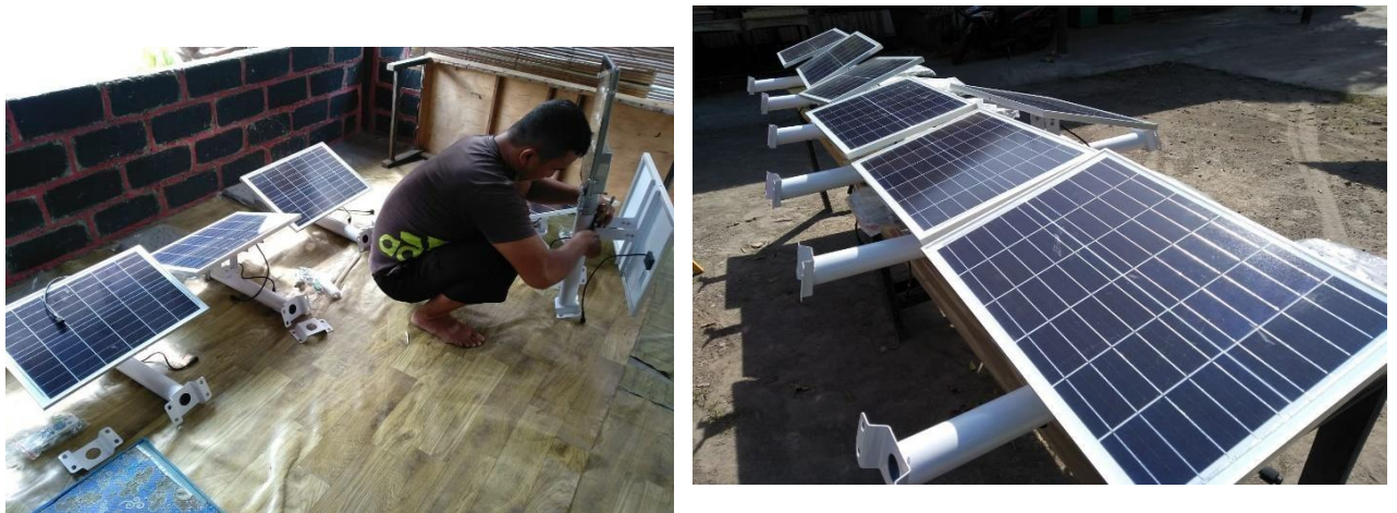
Gambar 4 instalasi panel surya
